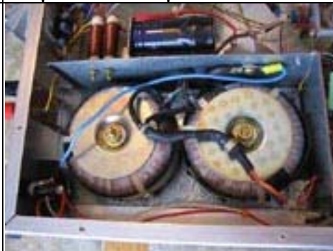
View of the toroidal transformers. The secondary taps of these, when rectified and filtered, provide the +35V and -35V DC power. I surrounded this power section with a grounded shield of galvanized sheet steel to protect the audio circuitry from EMI.
