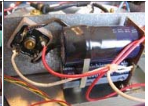
10A Bridge rectifier and filter capacitors for the DC power supply. The solid-state amplifiers do not require regulated DC. However, the DC supplies should be well-filtered to minimize line-frequency noise.
