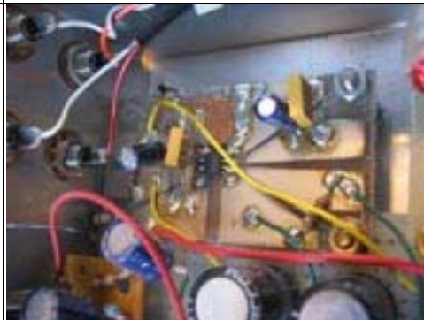
The LM4880 headphone amplifier circuit. The circuit board is DIY, etched from a small piece of copper-clad board. As is the case with the power amp, it's also important to cluster the components close to the IC here.
